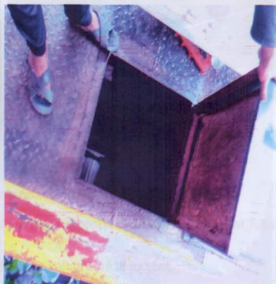
Fig B: Storage tank manhole/leak point
